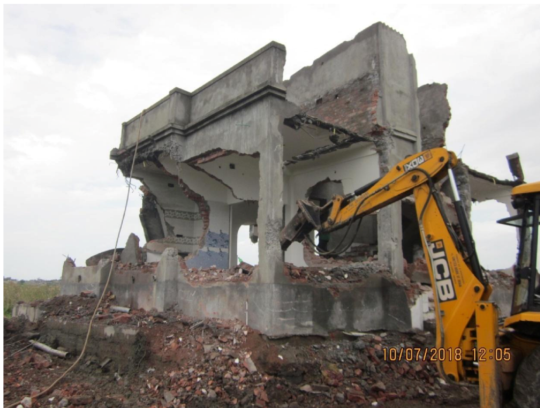
Picture 17. Demolition of illegal structures in East Kolkata Wetlands is a major task of the Authority
